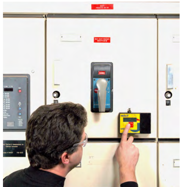
Figure 47, Photo Showing etd Mounted Outside of a Breaker Cubicle
